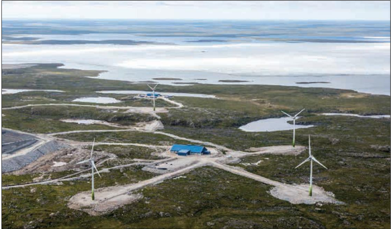
Photo 4.2-1: The Diavik 9.2 megawatt wind farm. The wind farm consists of four wind turbines.
